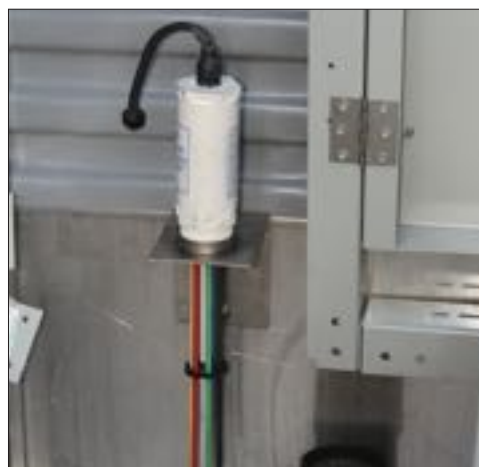
Electric Water Level Control
