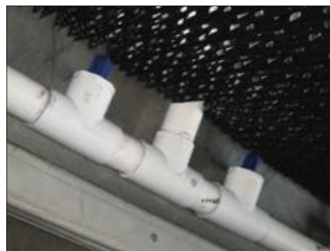
Basin Sweeper Piping
